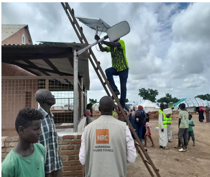
Picture 1: NRC, Installation of solar light unit at Al huri site, Gedaref.
