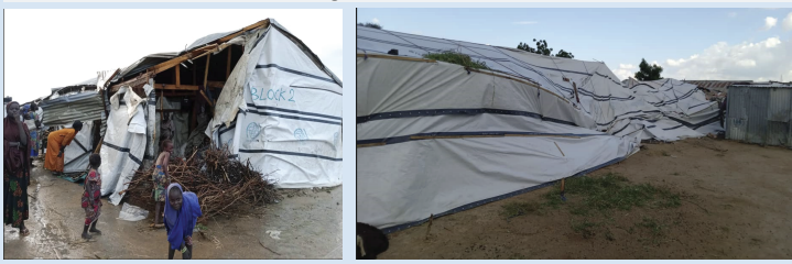
Pulka reception centre requires reconstruction with semi-permanent structure ©IOM
